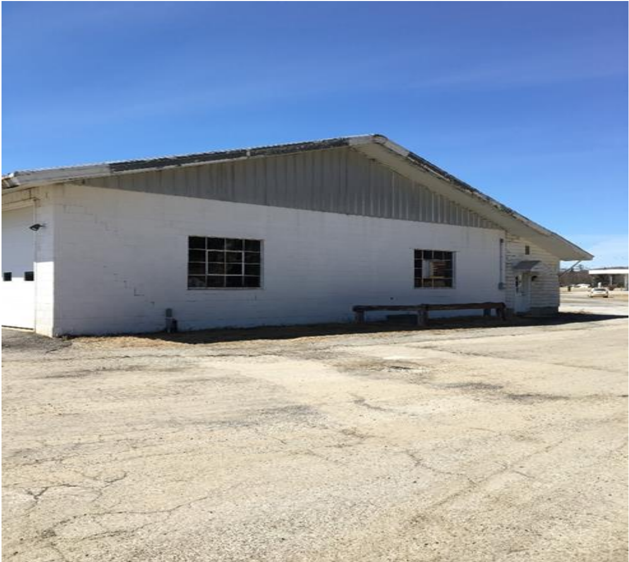
Rear view of existing building. Note deteriorated condition, single pane windows, rotten trim and cracks in uninsulated cinder block walls.
