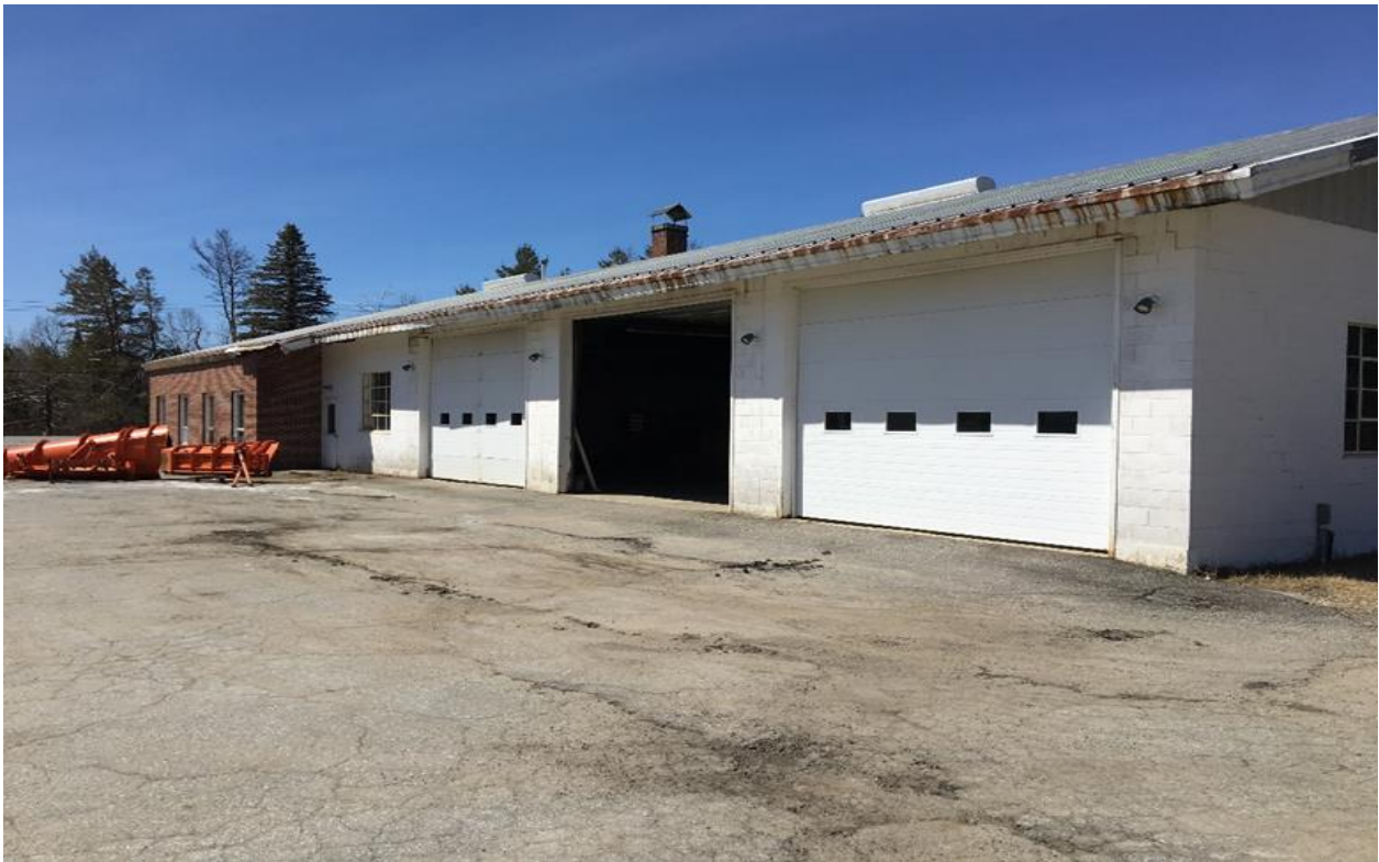
Rear right side view of existing building. Siding and building trim in need of replacement. Note holes in roof trim where pigeons and animals have access to shed interior. Also, shed end of roof is too low for building extension to increase storage or headroom inside the building.
