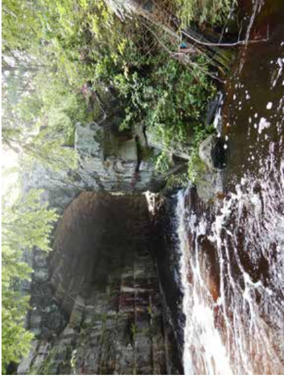
Concord-Lincoln Corridor, Concord Bridge #C5.20 Failing S.E. Dry Laid Stone Wing
