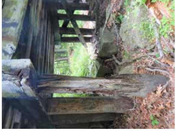
Concord-Lincoln Corridor, Woodstock Bridge #P18.17 Deteriorated Timber Bent Post
