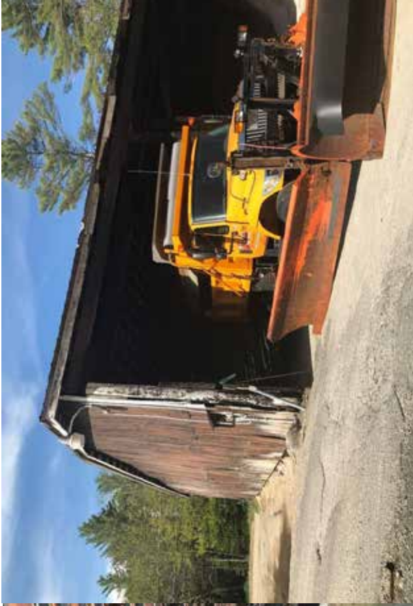
Lempster (215) – Salt Shed deteriorated condition
