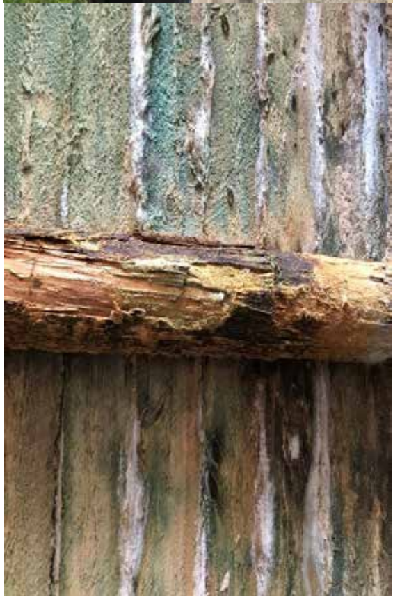
North Hampton (612) – Wall and post rot
