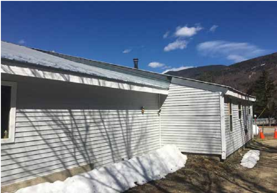
Rear view of existing patrol shed. Siding and building trim in need of replacement. Shed end of roof is too low for building extension to increase storage or headroom inside the building.
