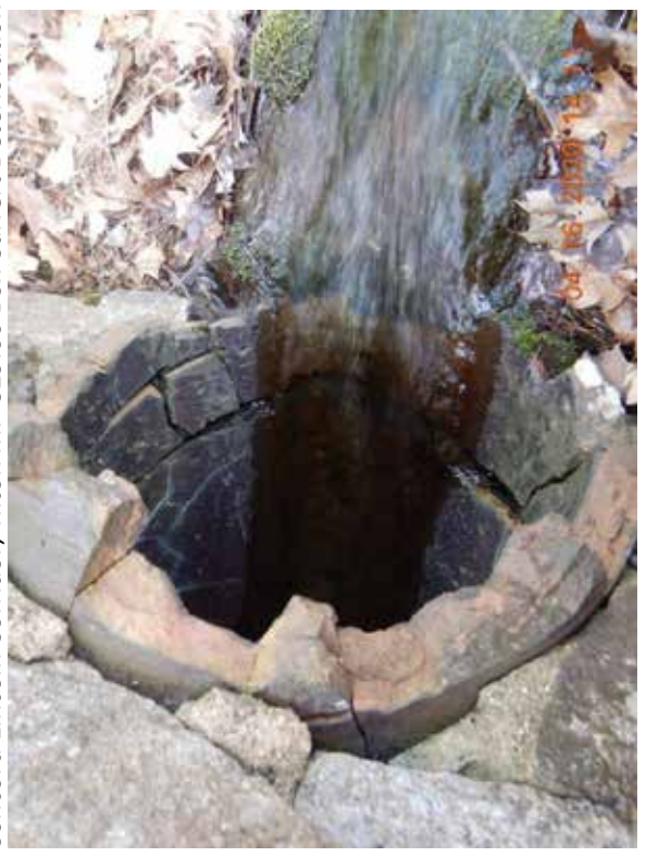
Concord-Lincoln Corridor, Laconia MP C34.91 Pipe Failure
