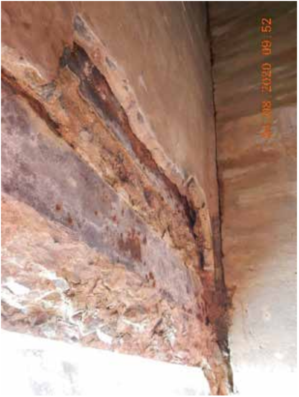
Concord-Lincoln Corridor, Tilton MP C19.66 Box Culvert Deterioration
