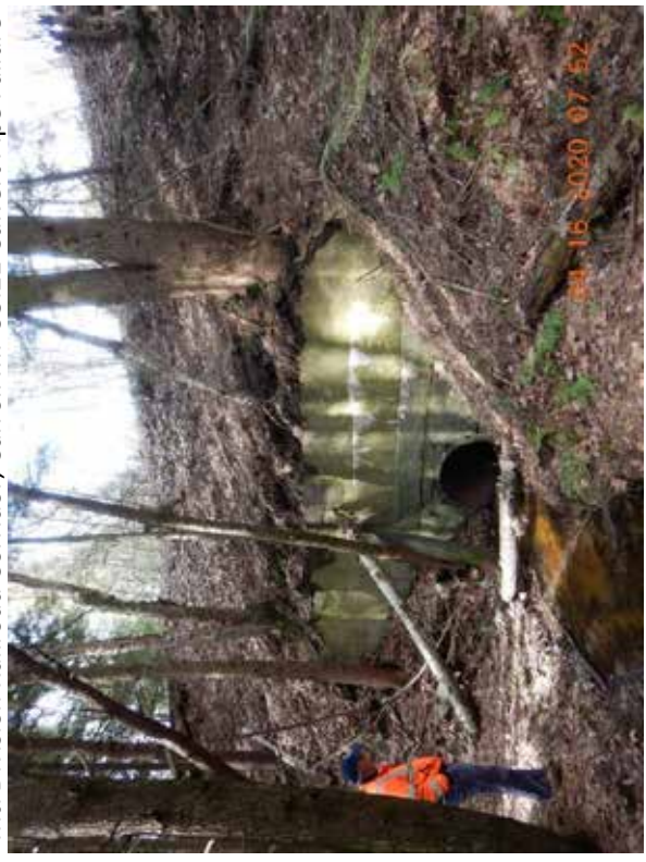
Concord-Lincoln Corridor, Canterbury Culvert MP C7.22 Vegetation Removal Required to Preserve Culvert Pipe Headwall Slope Retaining Structure
