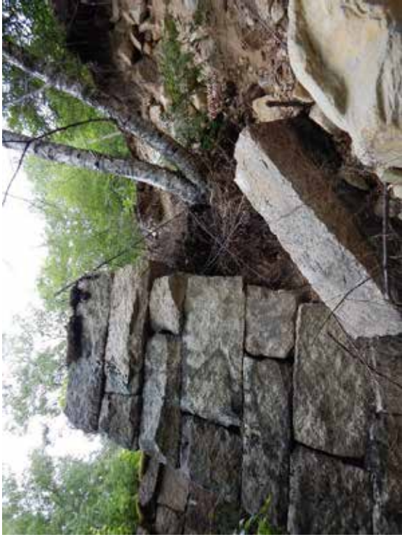
Mtn. Division Railroad Corridor, Harts Location Bridge #81.82 Failing N.E. Wing Slope
